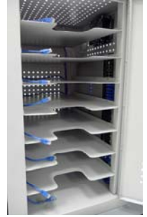
Cisco 24 port switch mounted internally
