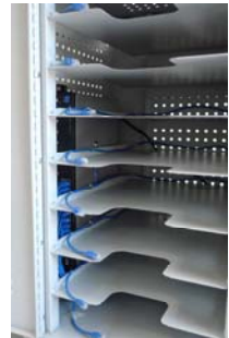
Cisco 24 port switch mounted internally
