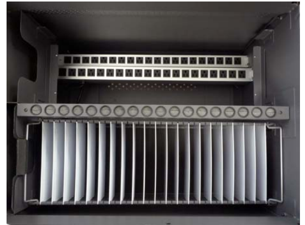
40 outlets positioned under trays
