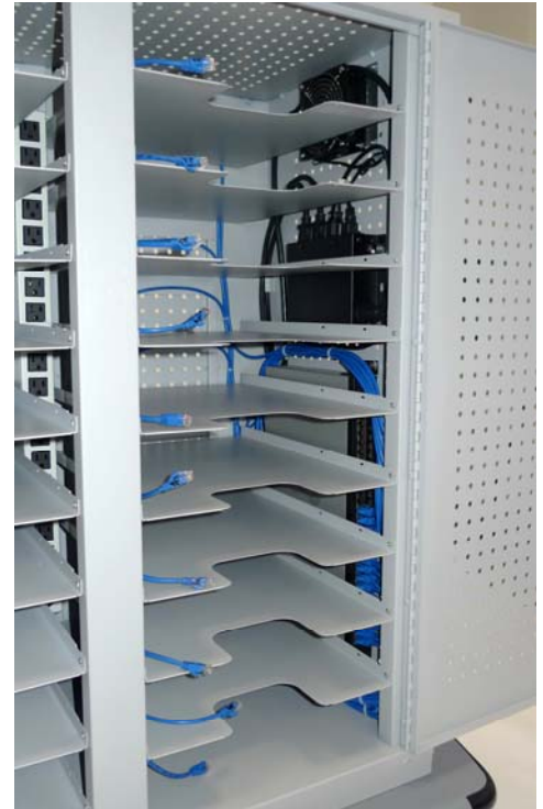
Fan, electronic switching timer, 48 port network switch and Ethernet cables all pre-installed
